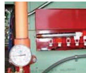
Spare Sprinkler Head Box
